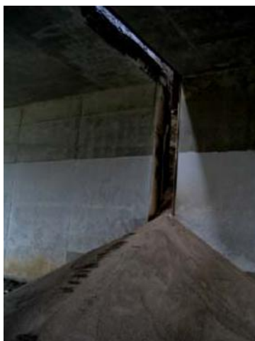
Fig 10-2. The gap in the culvert with square cross section due to earthquake
