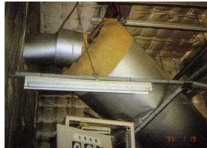
Fig. 9-5 Damage to sound-proof element
