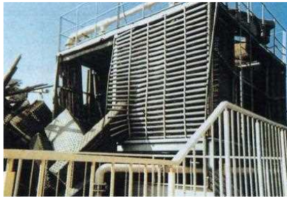
Fig. 9-2 Damage to cooling tower. No slide is reported due to existence of fillers (structures).
