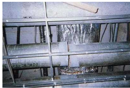
Fig. 9-3 Damage to piping of water cooling system (Due to lateral seismic force, the welded part of pipe has damaged)
