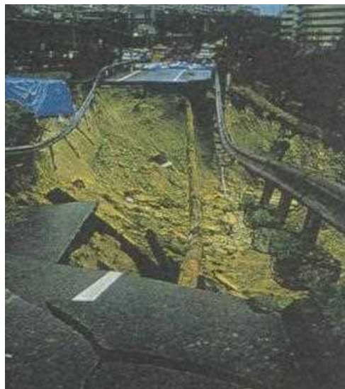
Figure 8-1 large scale ground movement due to landslide
