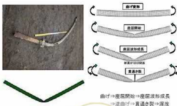
Figure 8-2 deformed pipe in landslide
