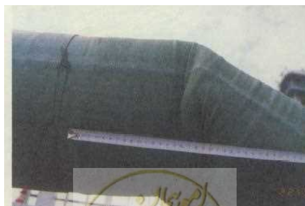
Figure 7-1 Cracks and buckling in bent pipe
