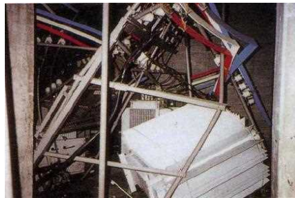
Fig. 9-7 Transformer has over turned in open air electric facilities' site
