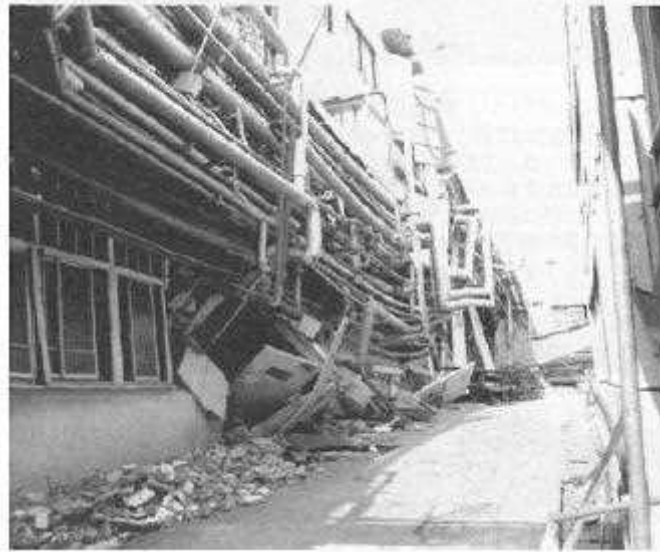
Figure 5-4 Damage to piping system due to damage to building
