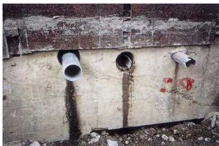
Fig. 9-4 Piping in the building inlet
