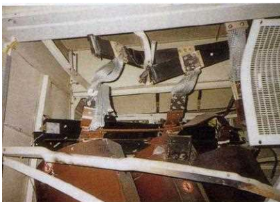
Fig. 9-8 Damage to transformer and its elements
