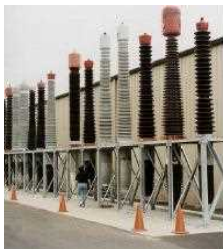
Figure 5-12: Bracing spare equipments in warehouse
