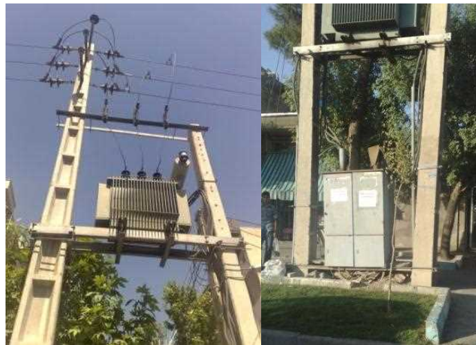
Figure 5-14: Distribution supports and aerial transformer
