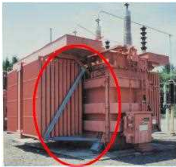
Figure 5-5: Reinforcing bracing of transformer's radiator
