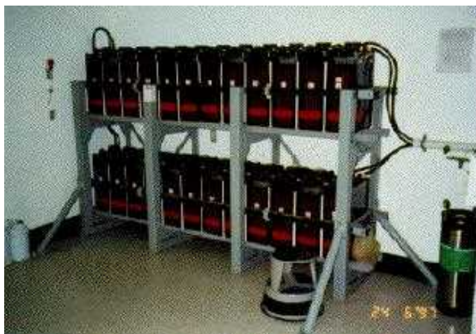
Figure 5-10: Batteries shelf bracing for controlling overturn
