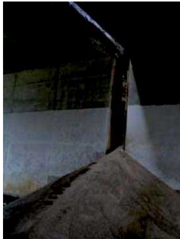
Figure 5-62 Crevice in Concrete Duct with Square Section due to Earthquake
