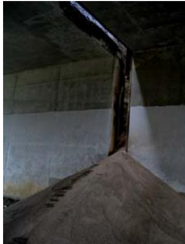
Figure 5.73. Gap in Concrete Conduit with Square Section due to Earthquake
